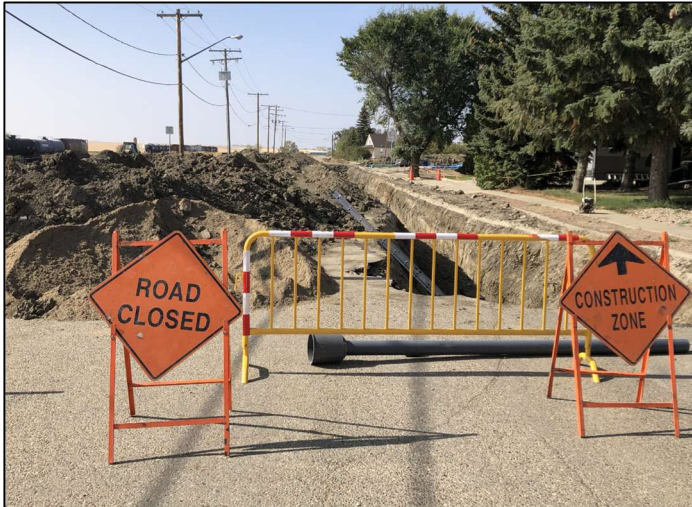
Figure 6 Break Evidence on 1st Avenue & 7 th Street
